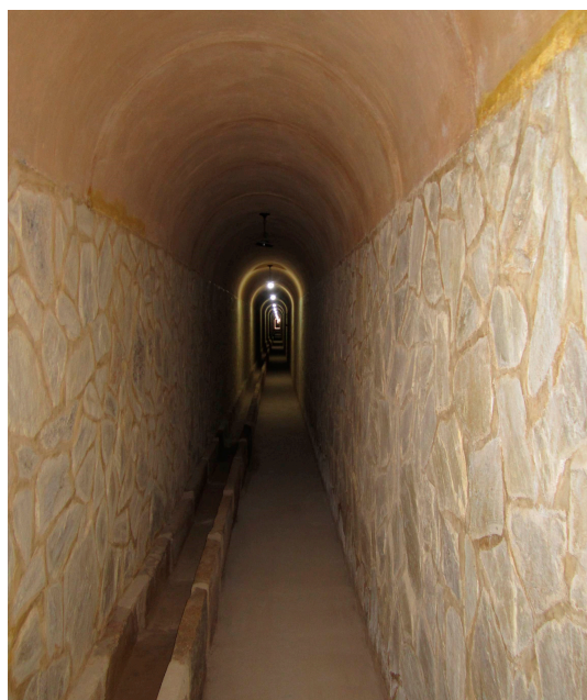
Figure 7. Rehabilitation of one of the mined mounds of the Irrigation Community of Cañada del Judío in Jumilla. Source: Authors (2 December 2022).
